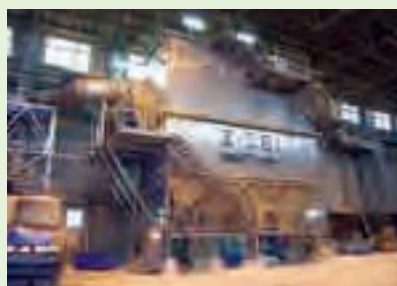
Phosphorus recovery facility of the dryer at the Chemical Fertilizer Plant (bug filter)
