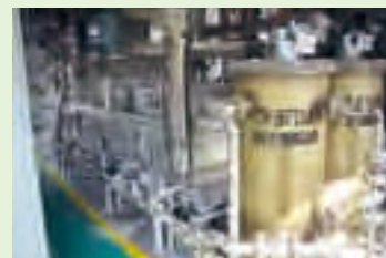
Vinyl chloride wastewater aggregators
