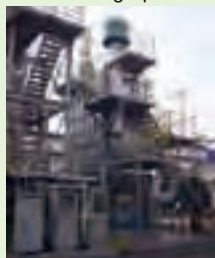
Exhaust gas incineration facility at the nitrobenzene plant
